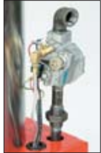
Elevated electronic gas control.
